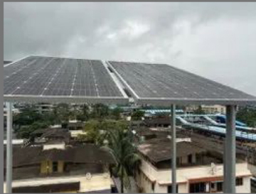
Residential Solar Panel Installation Service
